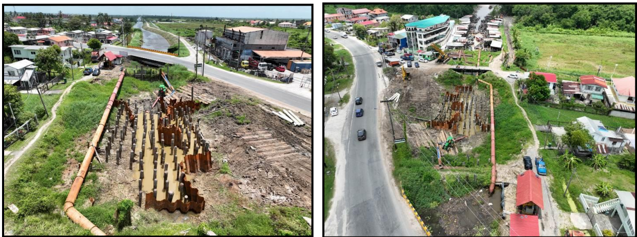
Photographs of the Pump Station at A- Line Sluice at Versailles – 22 August 2025
